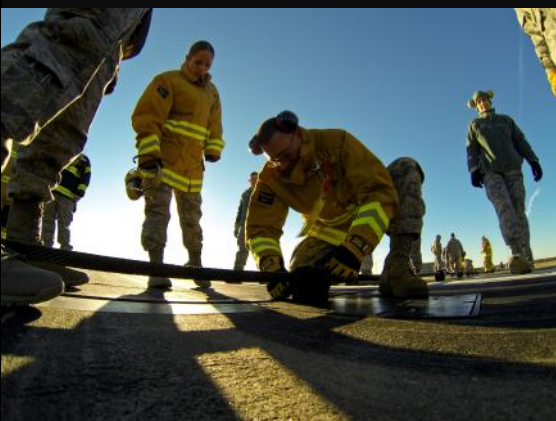
Airmen from the 177th Fighter Wing reset a cable during a cable arrestor system exercise, Nov. 14, at Atlantic City International Airport, N.J. The system, which is tested once a year, can aid any tail hook equipped aircraft to stop safely in the event of a failure of the braking systems. (U.S. Air National Guard photo by Tech. Sgt. Matt Hecht)
