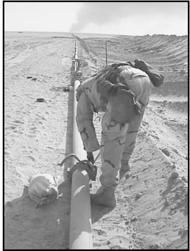
A soldier from the 62d Engineer Battalion couples a section of the pipeline while an oil fire burns in the background.
