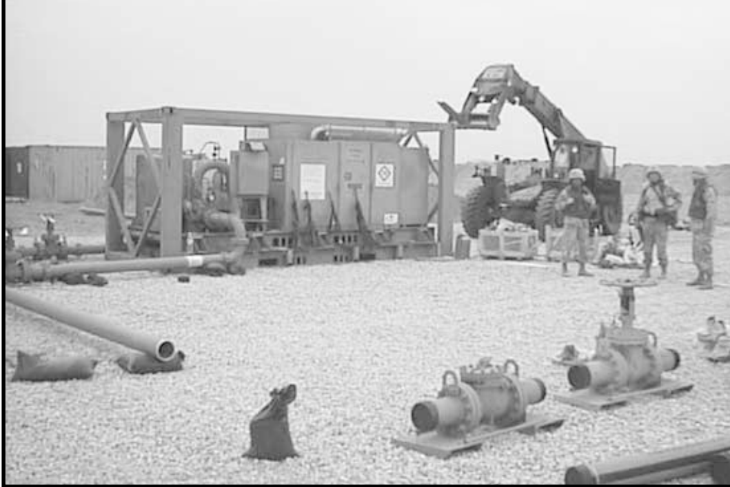
Soldiers from the 808th Engineer Company construct a pump station in Kuwait.
