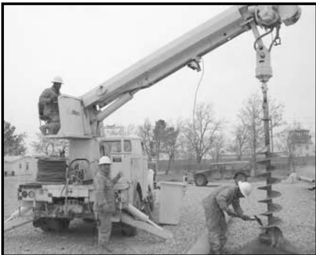
The crew sets a pole near the CJTF-180 building at Baghram Air Base, Afghanistan. A total of 130 45-foot concrete poles were set there by the 249th Engineer Battalion.
