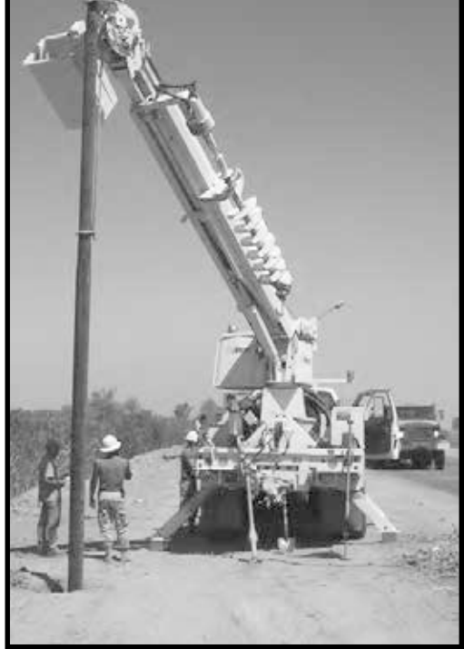
Soldiers from Bravo Company, 6th Platoon, 249th Engineer Battalion, erect a pole as they repair the high-voltage electrical system at Baghdad International Airport.
