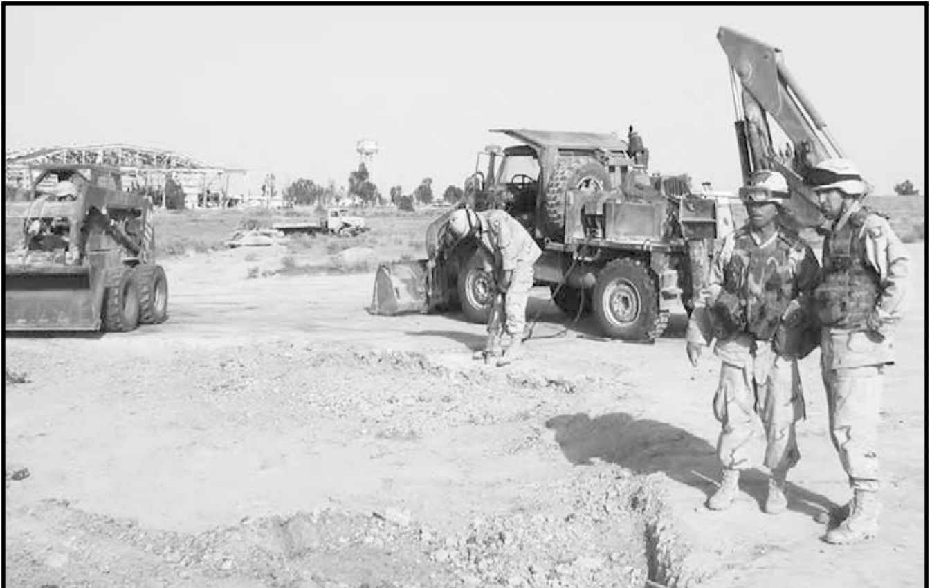
Soldiers from the 887th Engineer Company use a small emplacement excavator (SEE) and a Bobcat® to repair a crater in an airfield in northern Iraq.
