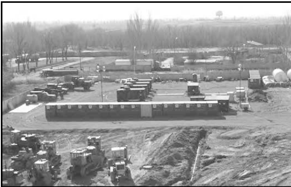
Power plant installed in Kyrgyzstan
