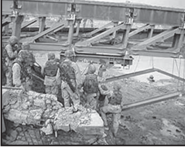
Army engineers installed two temporary bridges over the Khazir River on the highway between Mosul and Irbil. They were removed following repairs to the permanent bridge, which had been bombed during the fighting.
