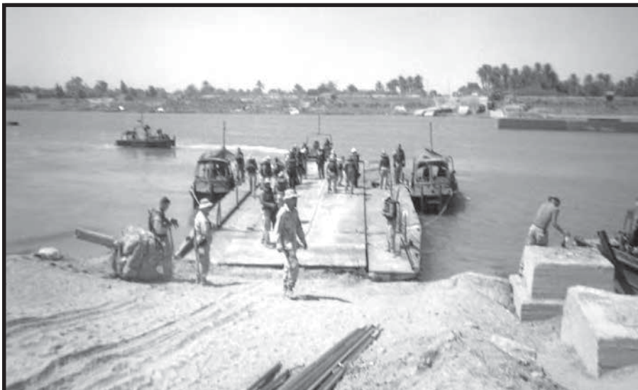
Military engineers from the Army, Navy, and Marine Corps begin construction on a float bridge across the Tigris River.
