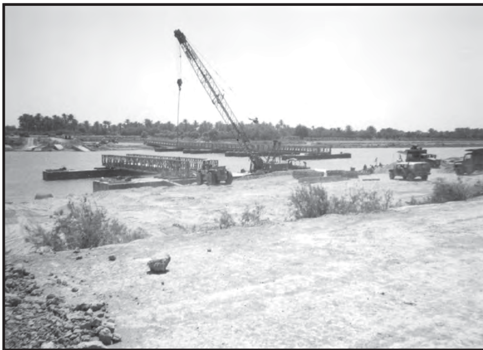
A Seabee crane helps attach a section of Mabey-Johnson bridge to a pontoon.
