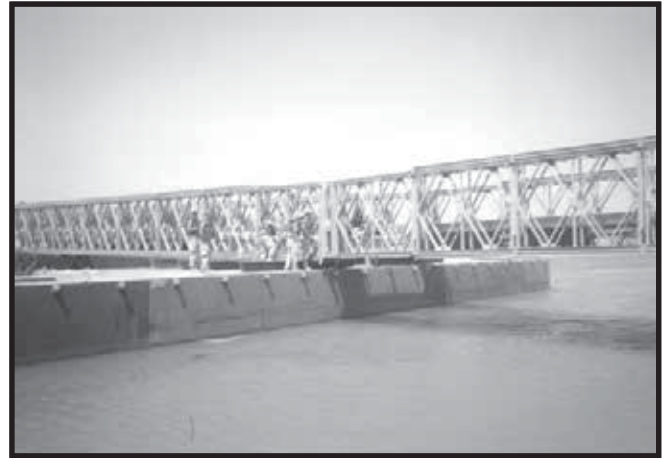
Engineers drive in the final pins to connect the near shore with the rest of the bridge.
