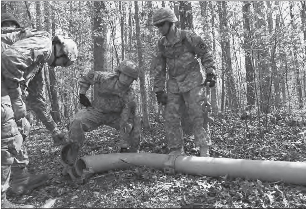
A Quartermaster Corps Soldier steadies a joint while it is clamped. Quartermaster Soldiers augmented the United States Army Reserve engineer units as needed throughout the exercise.
