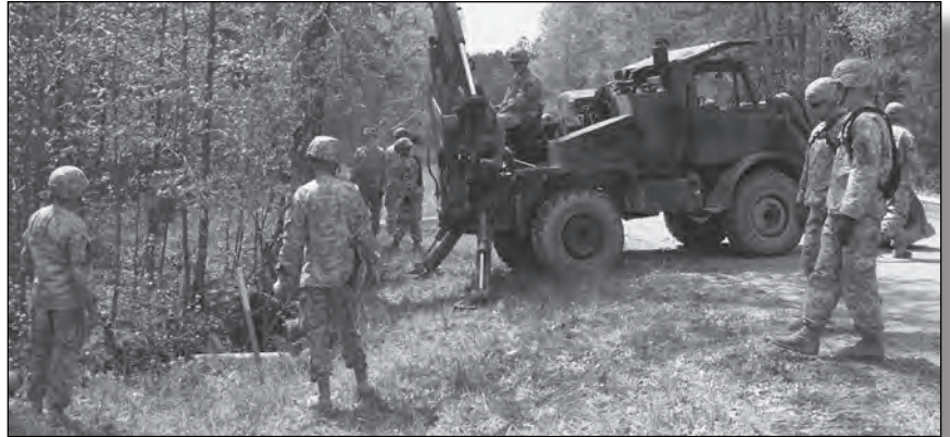
A small emplacement excavator pushes the pipeline through a culvert under a road.
