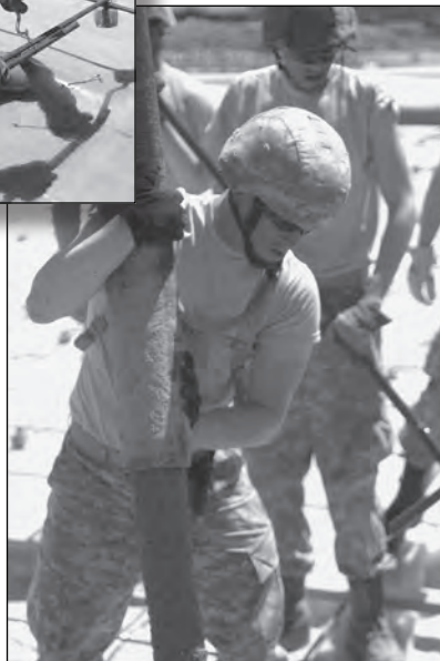
Left: A Soldier ties rebar stakes together with wire during the preparation for pouring a 102-by-82 foot pad.
