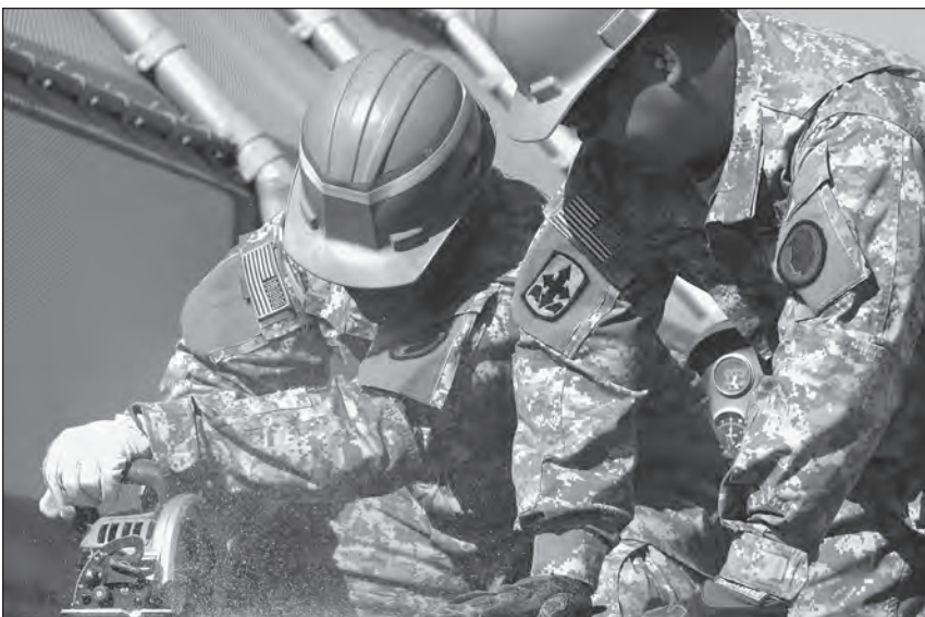
Soldiers build forms to surround electrical boxes and protect them from damage.
