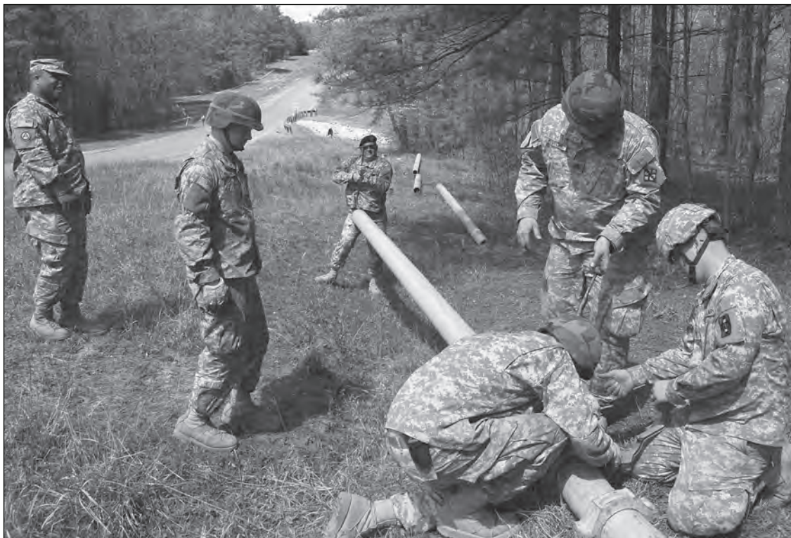
Engineers align the pipeline for clamping. The varying contours and elevations presented some challenges to Soldiers placing the pipeline.
