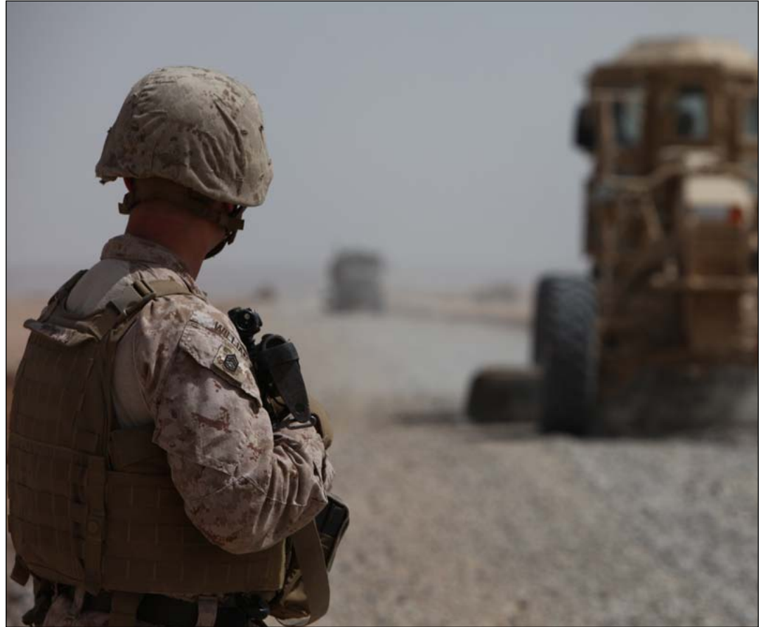
Gunnery Sgt. Joel Williams, heavy equipment chief, Heavy Equipment Platoon, Support Company, 9th Engineer Support Battalion, 1st Marine Logistics Group (Forward), watches while a grader levels the gravel during road construction outside of Forward Operating Base Geronimo, March 23.
