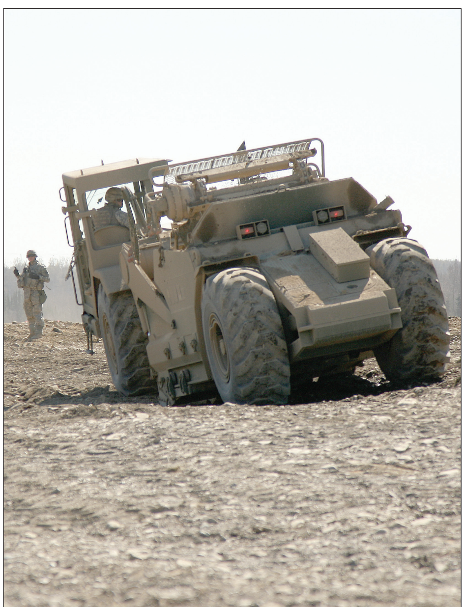
Soldiers of 84th Engineer Support Company dug up a 50 year-old concrete foundation at Camp Carroll, improved roadways at the Engineer Skills Training Area, and conducted terrain leveling operations at Bryant Army Airfield – a project scheduled to continue for the next several months. (Photo by Percy Jones/JBER PA)
