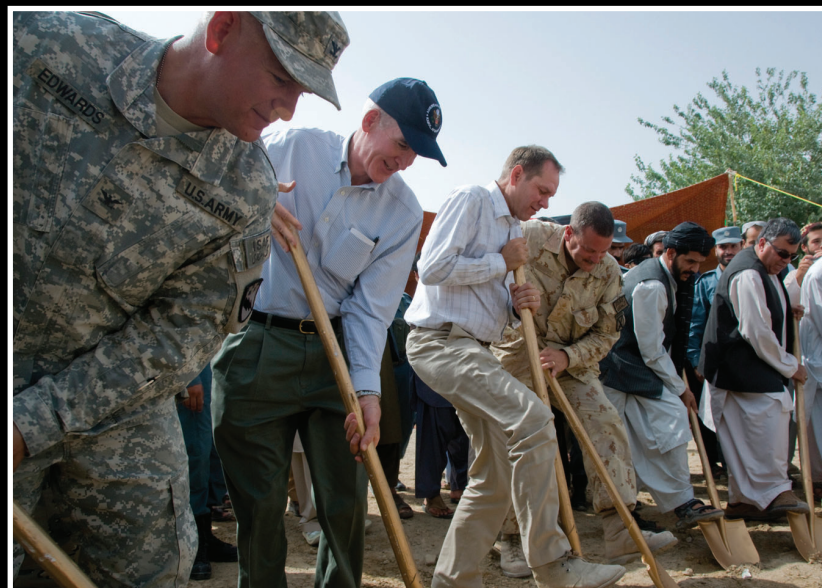
U.S. Army Col. James Edwards, commander, 525th Battlefield Surveillance Brigade, and representatives from the U.S. State Department, Canada and the Weesh District government, break ground for the customs depot expansion project in Weesh July 6. (Photo by U.S. Air Force Senior Airman Jessica Lockoski, 525th BfSB Public Affairs)
