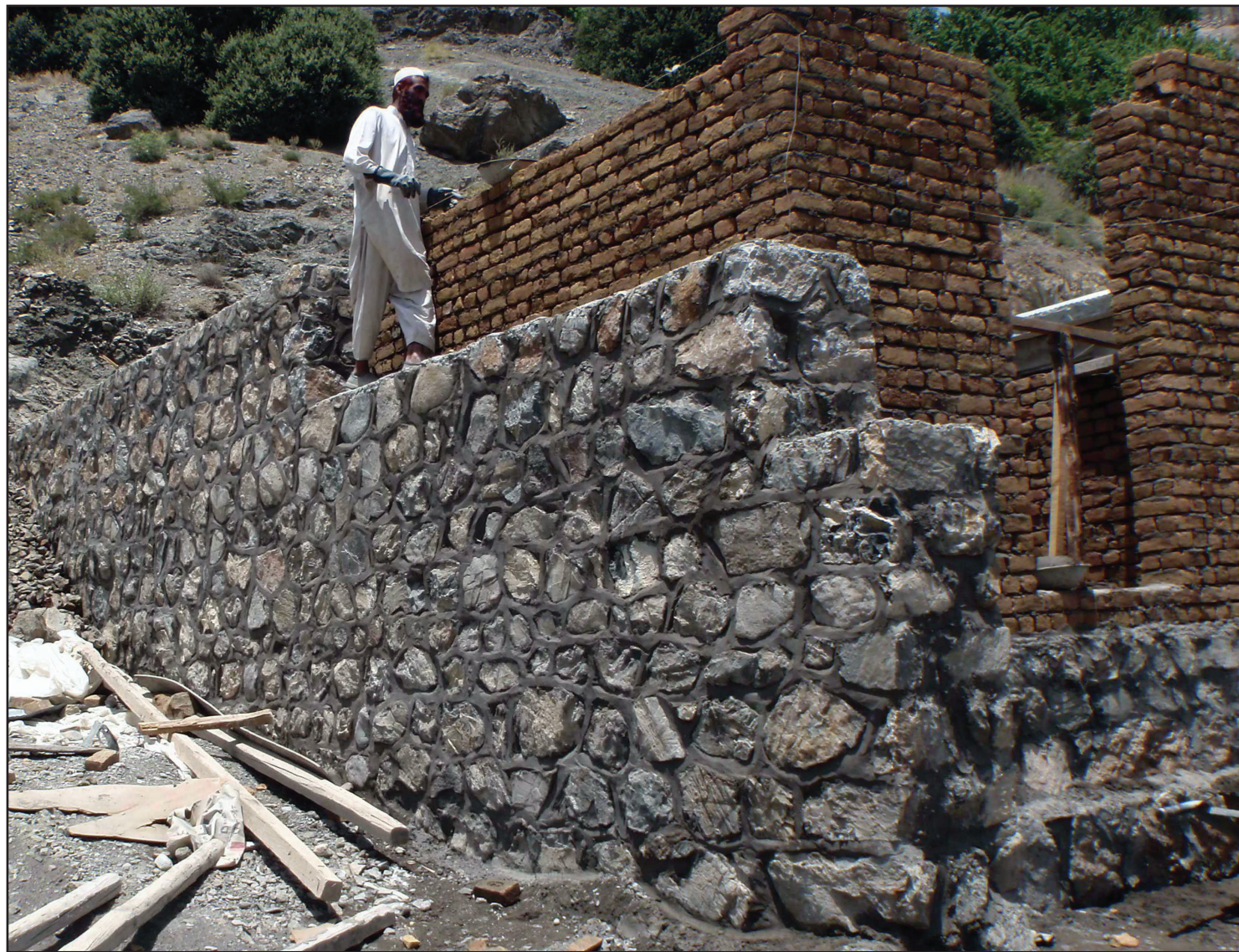
An Afghan construction worker lays bricks for the outer wall of the Showat basic health clinic July 12. The project was submitted through the Paktya Provincial Development Plan and is scheduled to open this August. (Photo by U.S. Air Force 1st Lt. Cale Reeves, Paktya Provincial Reconstruction Team)
