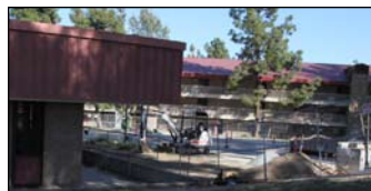
Construction on an outdoor fitness area recently began on the 14 Area gym.
