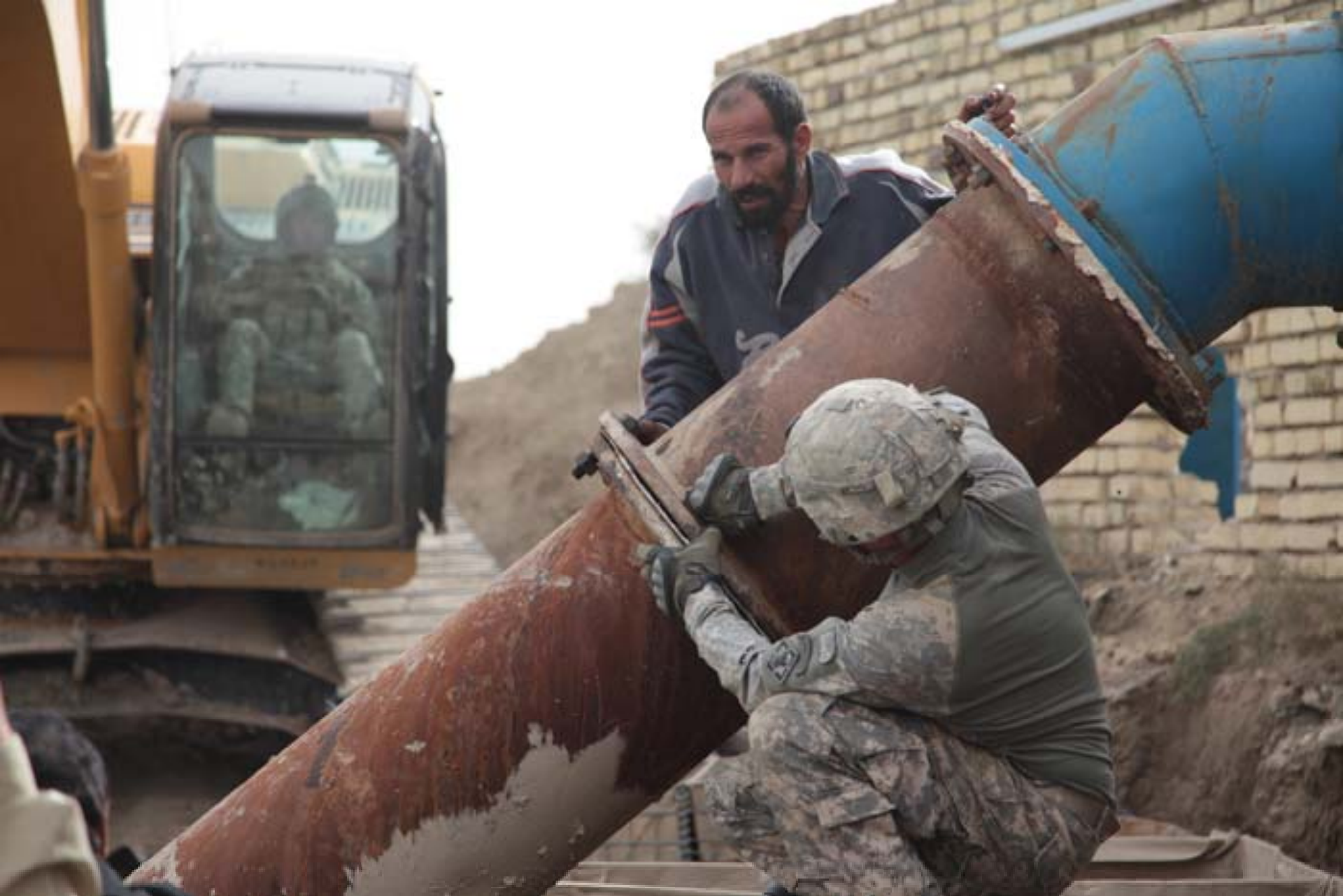
U.S. Soldiers, assigned to 194th Engineering Brigade, and local a man attach a pipe while repairing a water main in Al Batha, Dhi Qar, Iraq, January 18, 2010. (U.S. Army photo by Specialist Ernest E. Sivia III/Released) 100118-A-9234S-079
