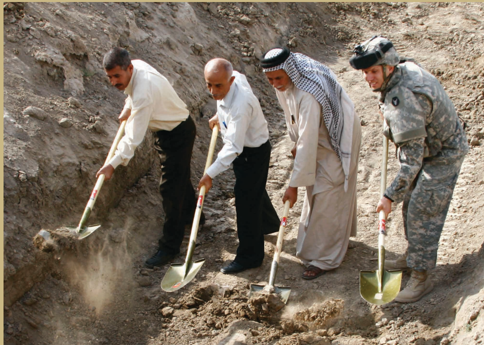
Engineer Talib Harigeh, (left) Engineer Reishan Shanwah Juwaid, City Councilman and Sheik Mohammed Al Tayeh, and Capt. Andrew Peterson break ground on Task Force WOLVERINE's agriculture project. Photo by Maj. Scott Ebel, Task Force WOLVERINE UPAR.
