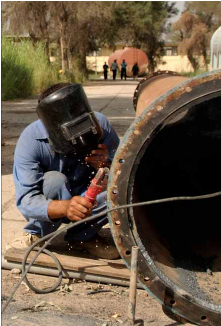
BAGHDAD – An Iraqi laborer welds water pipes used in water treatment facilities in Baghdad's International Zone. The projects of the 4th Brigade Combat Team's Special Troops Battalion's Infrastructure Coordination Element provide both temporary and permanent employment to Iraqis and, in most cases, the Iraqi contractors hire local laborers from the different districts where the projects take place, said Capt. Ryan Parks, sewer and water projects manager, STB, 4th BCT, 4th Infantry Division.
