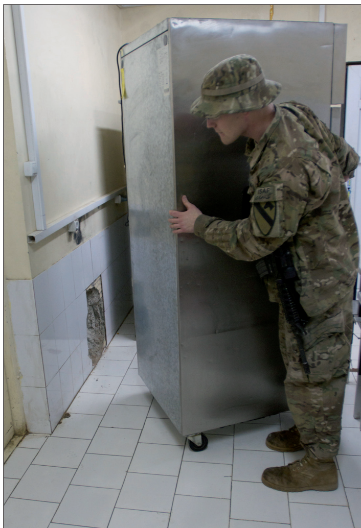
U.S. Army Spc. James Young, a native of Coquille, Ore., moves a refrigerator to expose the hole on the wall one of three rockets made on December 23, 2012, at the dining facility Forward Operating Base Naghlu High. Young serves as a food service specialist assigned to Headquarters and Headquarters Company, 2nd Battalion, 7th Cavalry Regiment, 4th Brigade Combat Team, 1st Cavalry Division based out of Fort Hood, Texas. (U.S. Army photo by Staff Sgt. Richard Andrade, Task Force Long Knife Public Affairs)
