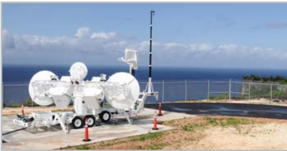
This Joint Threat Emitter satellite provides an electronic signal to aircraft, at Ritidian Point on Northwest Field, Guam, Jan. 29, 2013. The Air Force and Navy radar and satellite systems, known as the JTE, provide ground threat warnings up to the aircraft to simulate an attack, improving Andersen's operational readiness. (U.S. Air Force photo by Airman 1st Class Mariah Haddenham/Released)
