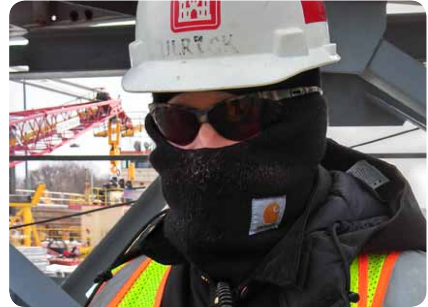
Jim Ulrick, operations, works on the Lock and Dam 6 dewatering project, near Trempealeau, Wis., Feb. 19.
