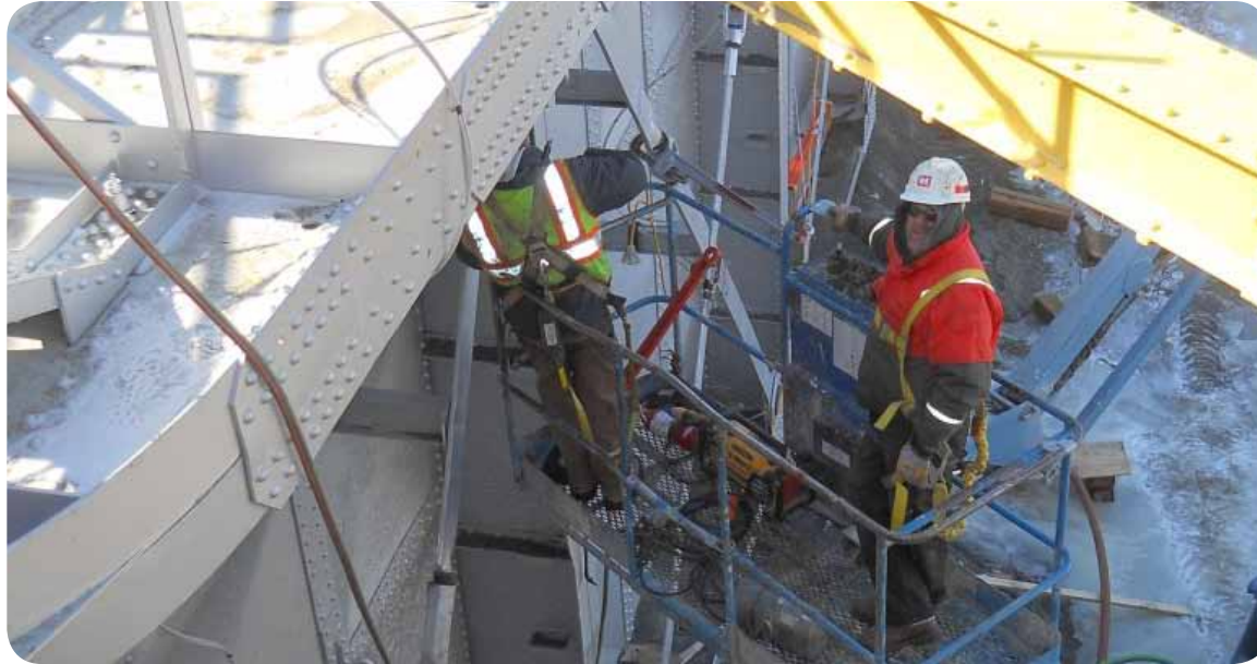
Chad Anderson, operations, left, and Joseph Lakey, operations, work on repairing the diagonals on one of four gates at Lock and Dam 6, near Trempealeau, Wis., Feb. 19.
