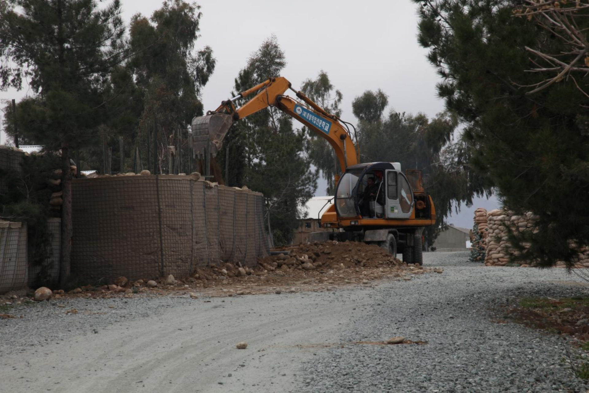
An Afghan local national uses a machine to load dirt into Hesco barriers on Forward Operating Base Mehtar Lam, Laghman province, Afghanistan, Feb. 25, 2013. The newly erected barriers are to section off the side of the base that has recently been turned over to the Afghans. (U.S. Army photo by Spc. Andrew Claire Baker/Released)
