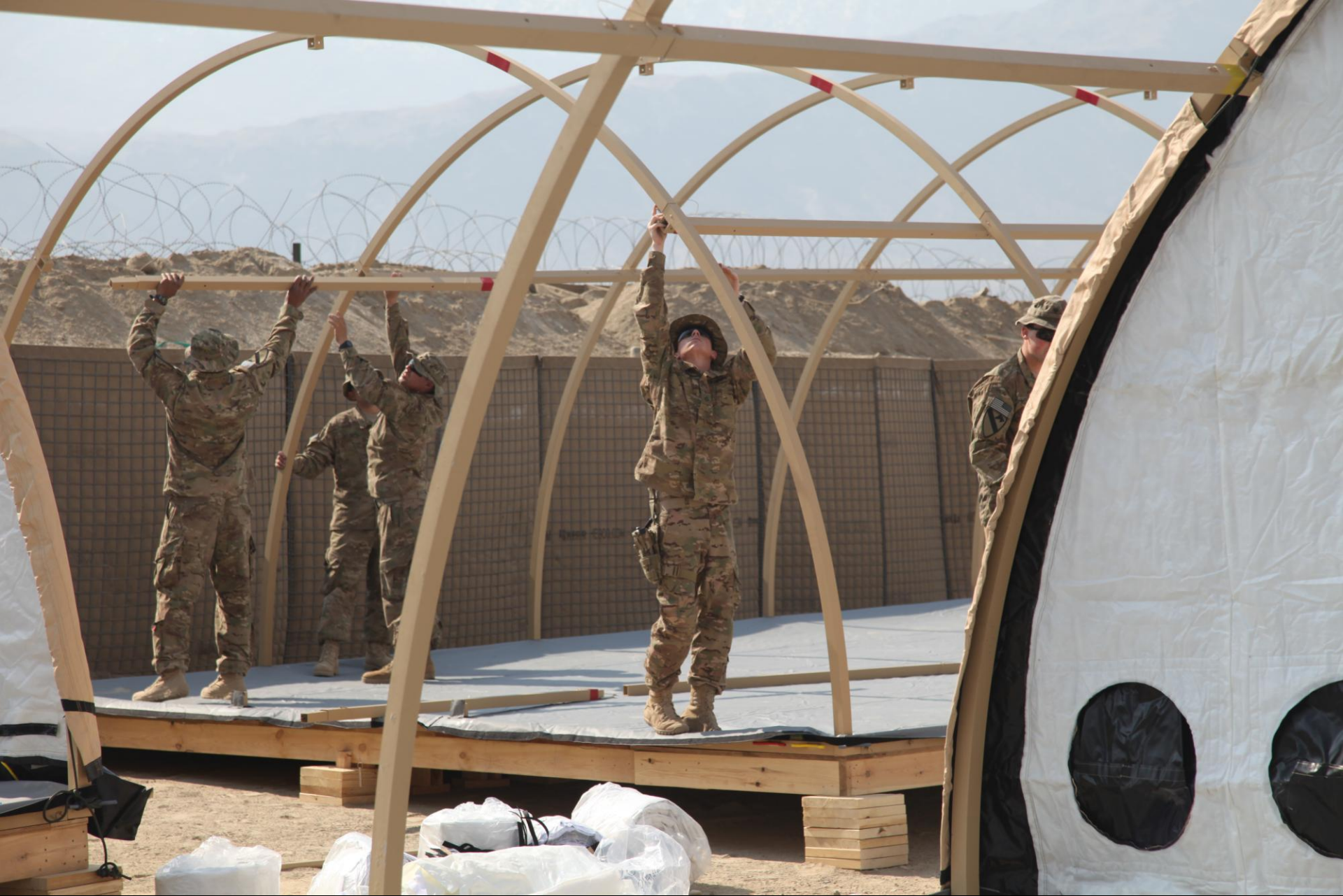
U.S. Army Soldiers serving with 4th Brigade Special Troops Battalion, 4th Brigade Combat Team, 1st Cavalry Division construct new living quarters on Forward Operating Base Xio Haq, Laghman province, Afghanistan, Feb. 13, 2013. The Soldiers are constructing new living quarters for Soldiers coming from bases that will be shut down in the future. (U.S. Army photo by Spc. Andrew Claire Baker / Released)
