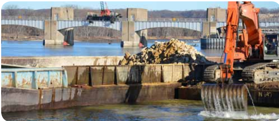
A construction worker removes rock from the Mississippi River during construction at Lock and Dam 3, near Red Wing, Minn., Jan. 10, 2012.
