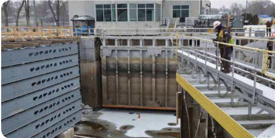
A district employee monitors work at the Lock and Dam 6 dewatering, near Trempealeau, Wis., Jan. 16. The lock is dewatered approximately every 20 years for maintenance.
