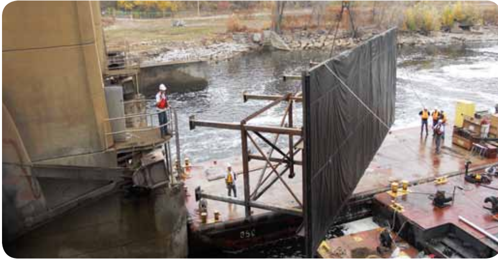
Maintenance and repair employees place a temporary dam, or cofferdam, on the Lower St. Anthony Falls Lock and Dam in Minneapolis during repairs Sept. 20, 2012.
