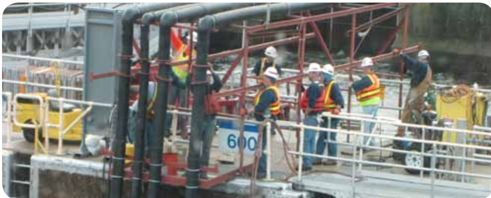
District staff begin preparing Lock and Dam 6, near Trempealeau, Wis., for dewatering in December 2012. The team is scheduled to be complete with the repairs around March 11.
