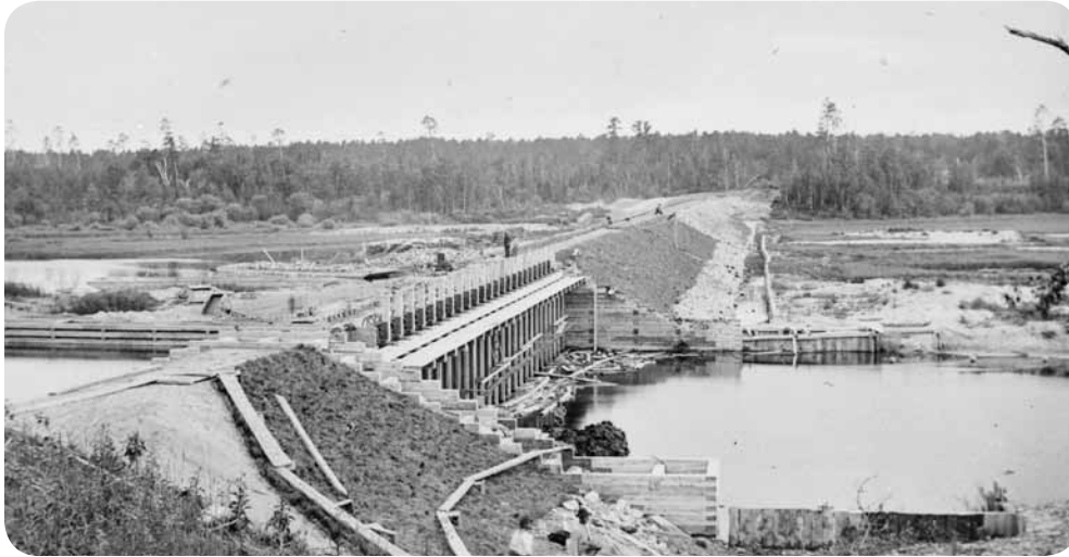
Corps of Engineers construction employees work on the Winnibigoshish Dam, near Deer River, Minn., in 1884. The Corps received $75,000 in 1880 to begin constructing the dam.
