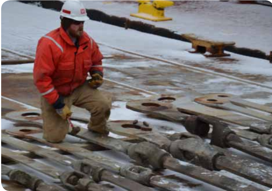
Brandon Olson, operations, works on diagonals for the Lock and Dam 6 lock gates during the dewatering at the Trempealeau, Wis., lock and dam. The project began Dec. 3, 2012.
