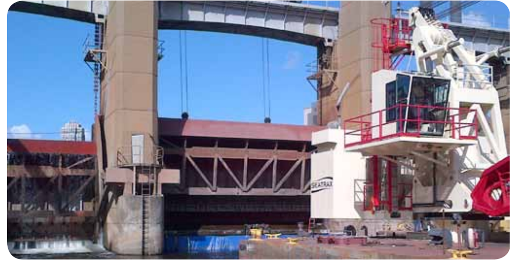
A barge from the maintenance and repair section in Fountain City, Wis., is used by district staff to complete concrete repairs to Lower St. Anthony Falls Lock and Dam in Minneapolis Sept. 20, 2012.
