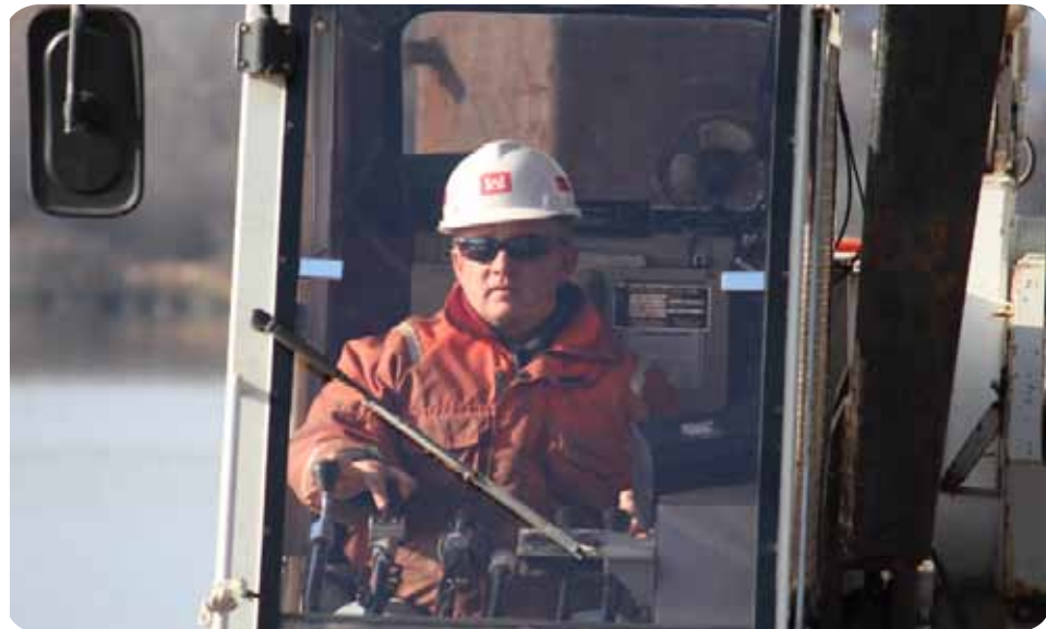
Knute Knutson, operations, operates a crane during work at the Lock and Dam 6 dewatering, near Trempealeau, Wis., Jan. 16.
