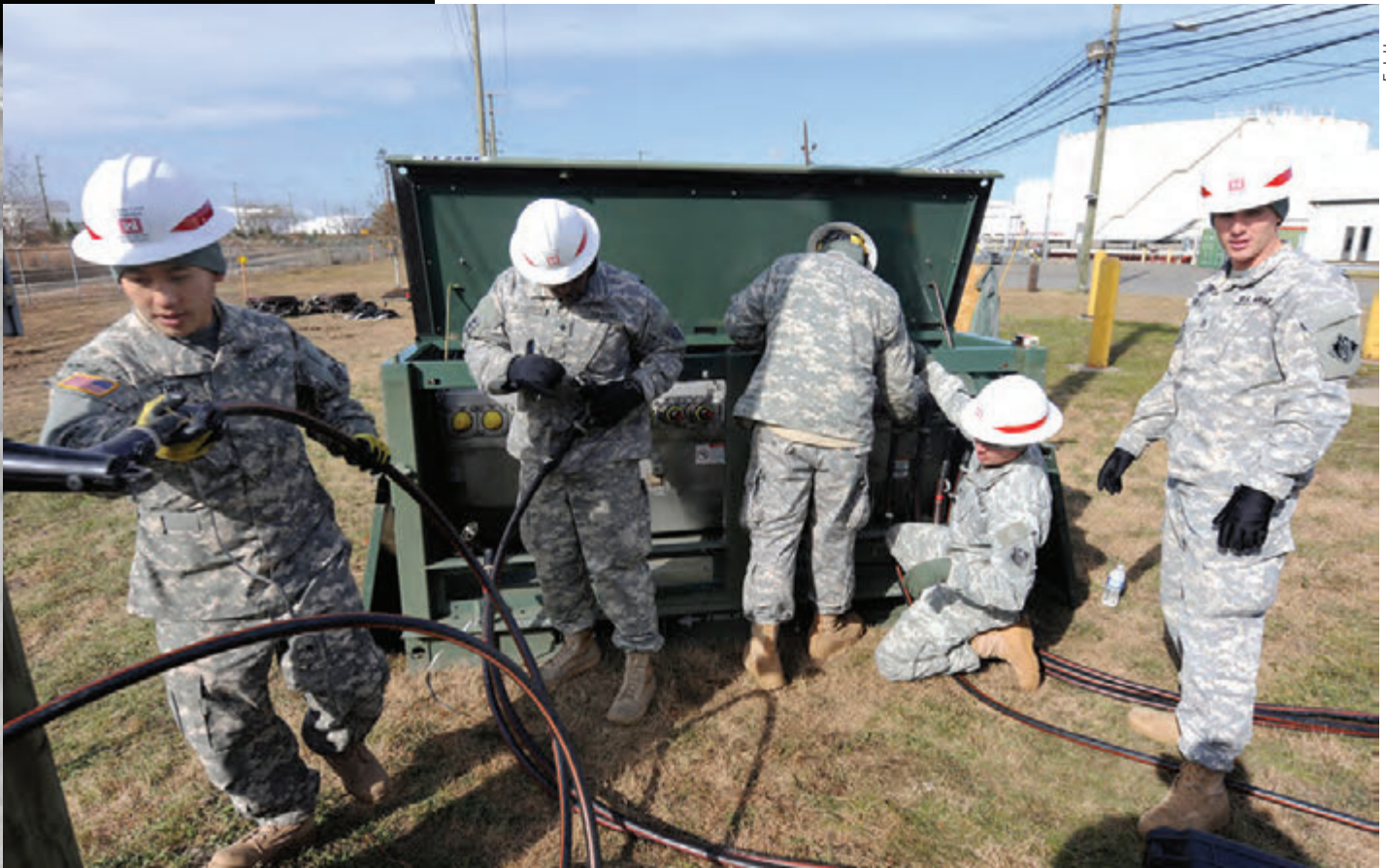
Soldiers install electrical generator equipment at a Carteret, N.J., fuel depot that lost power during Hurricane Sandy. DLA Energy provided fuel to state, local and federal responders for electric generators and water pumps.
