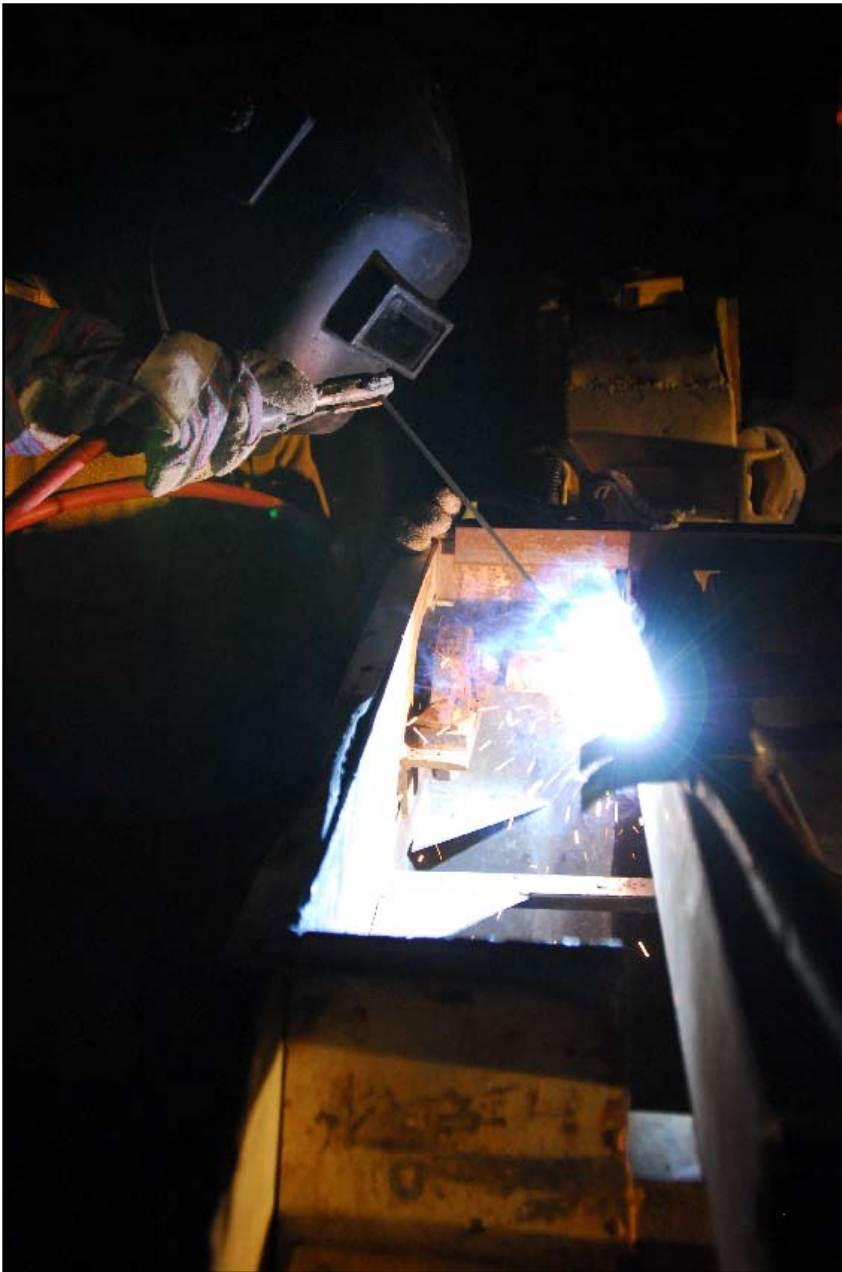
Dunga Katwal, welder, Fluor, makes emergency repair to a gate damaged when it was accidentally struck by a vehicle on Camp Victory Thursday.
